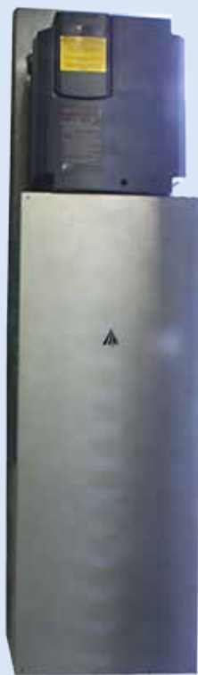
Drive mounted in shaft
