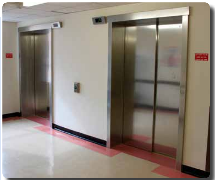
A typical hospital landing layout including landing doors, frames architraves, push buttons and LED indicators.
