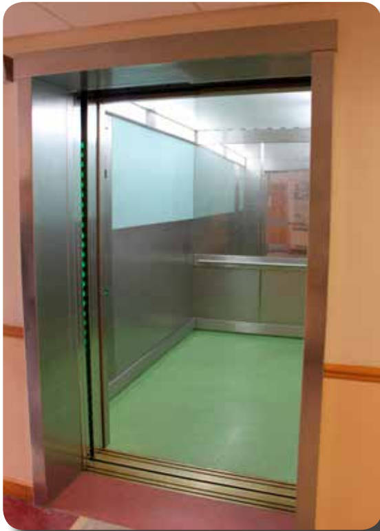
Typical hospital bed / passenger lift car with a combination of laminate and stainless steel finishes to the car walls.
